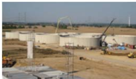
A total of five modules produce 10,000 m 3 biogas.
