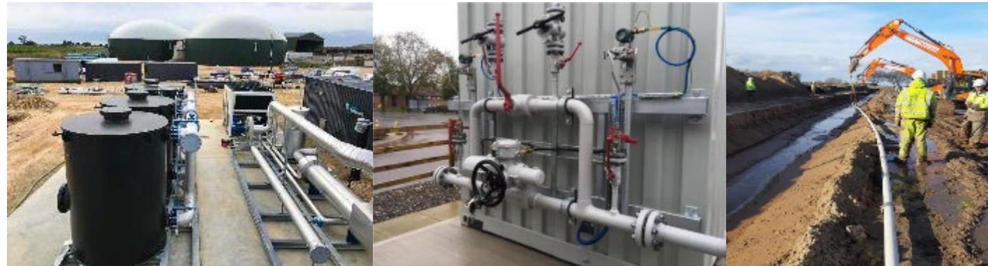
Photos from the first NTS Biomethane Injection Project at Somerset Farm Murrow Completed in 2020
