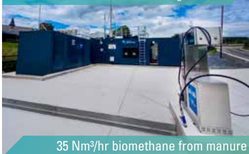
PurePac Mini with bio-CNG filling station
