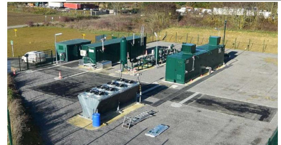
GrDF Reverse Flow station in France (7 bar to 50 bar)
