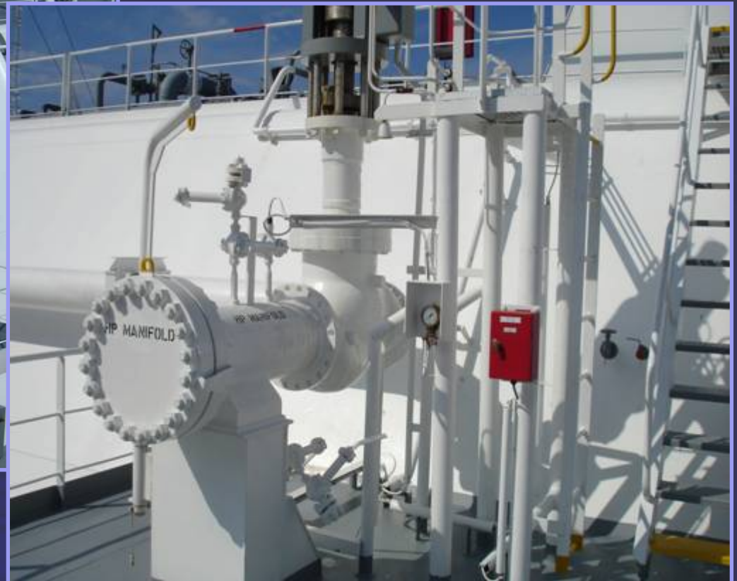
High Pressure Gas Manifold
