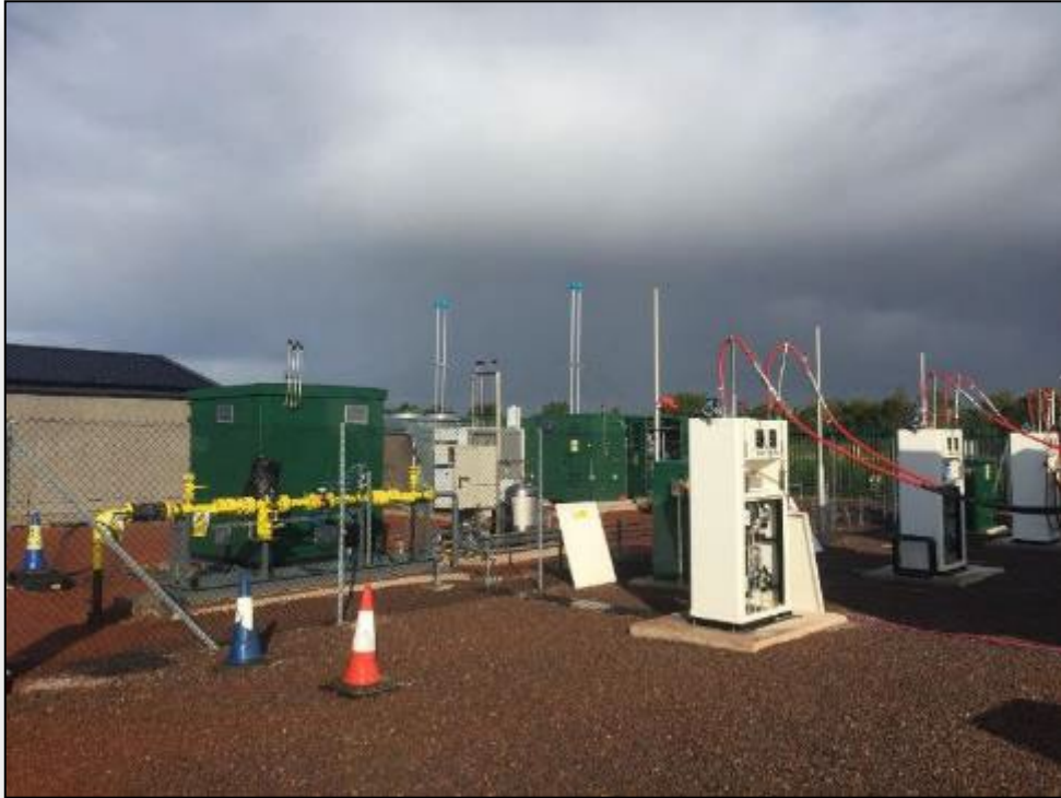
Meter, Odorant Unit, CV Measurement and Dispensers
